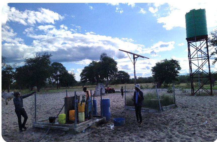
5-Solar powered borehole in Jamba-Luana
